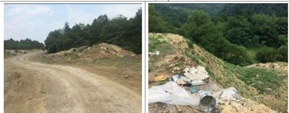
Figure 22. Deep cuts, trenches and pits, are without relevant barriers and warning signs
