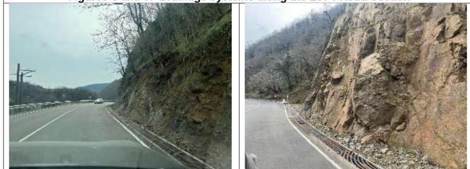
Figures 8 and 9: Drainage systems along the Lot 1 Road Section
